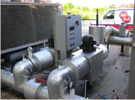
Pump retrofit complete. Two 10-hp pumps replace two 20-hp pumps which offer attractive savings.
